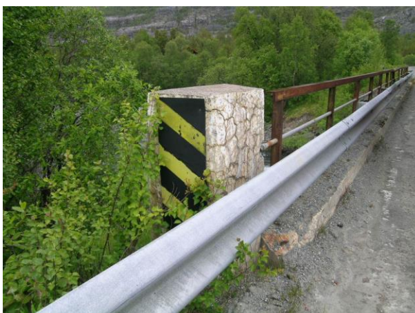
Figur 34 – Krakelert endestolpe i betong.
